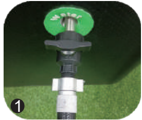
1 Close the valves of the inlet and outlet of the bathtub
